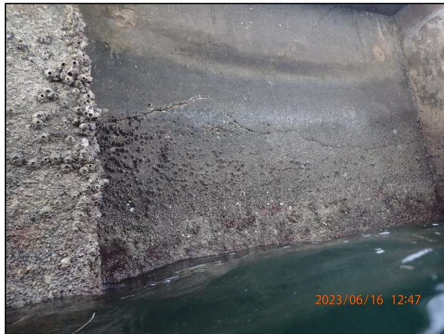
Photo 66: Typical 1/8 in. cracking of the concrete panels
