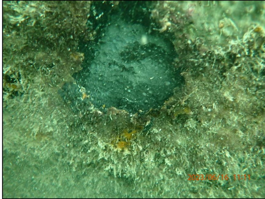
Photo 71: STA 12+18 Cleaned section of steel sheet pile for UTM reading with major to severe pitting
