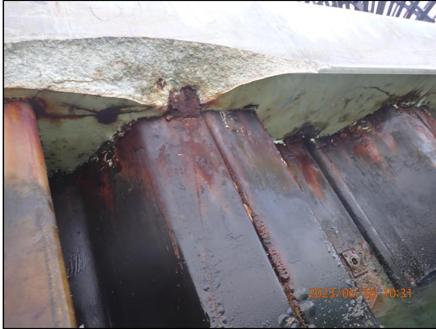
Photo 76: Localized major spalling with widespread cracking of the concrete cap
