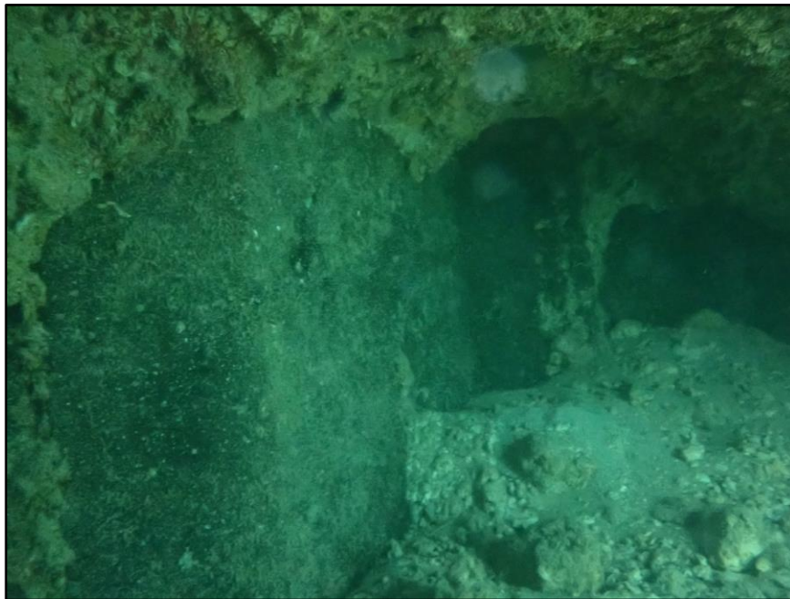
Photo 37: Section 12 View of new steel sheet pile portion of combi-wall through deterioration in original outer sheet
