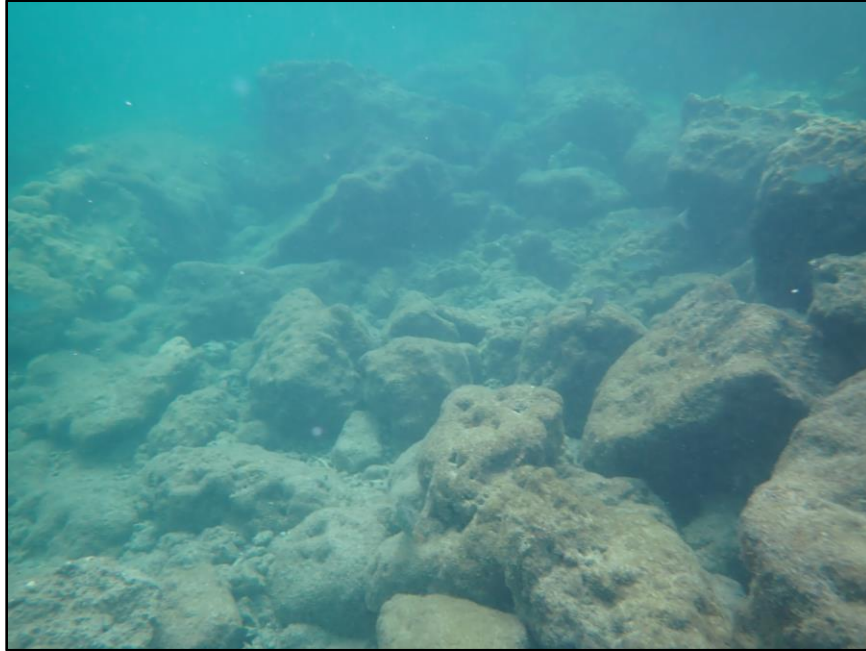
Photo 103: Below water riprap in line with above water steeper grades indicating movement of the stones from their original position
