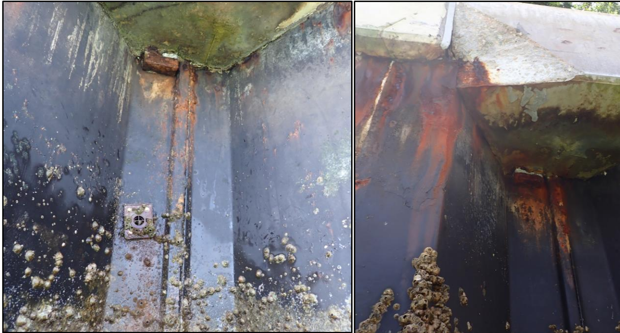
Photo 83: Typical condition of steel sheet pile STA 4+64 – STA 9+39 and major cap spill at STA 4+64
