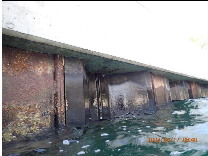
Photo 85: Minor corrosion of HZ piles and minor rust staining of AZ sheet pile
