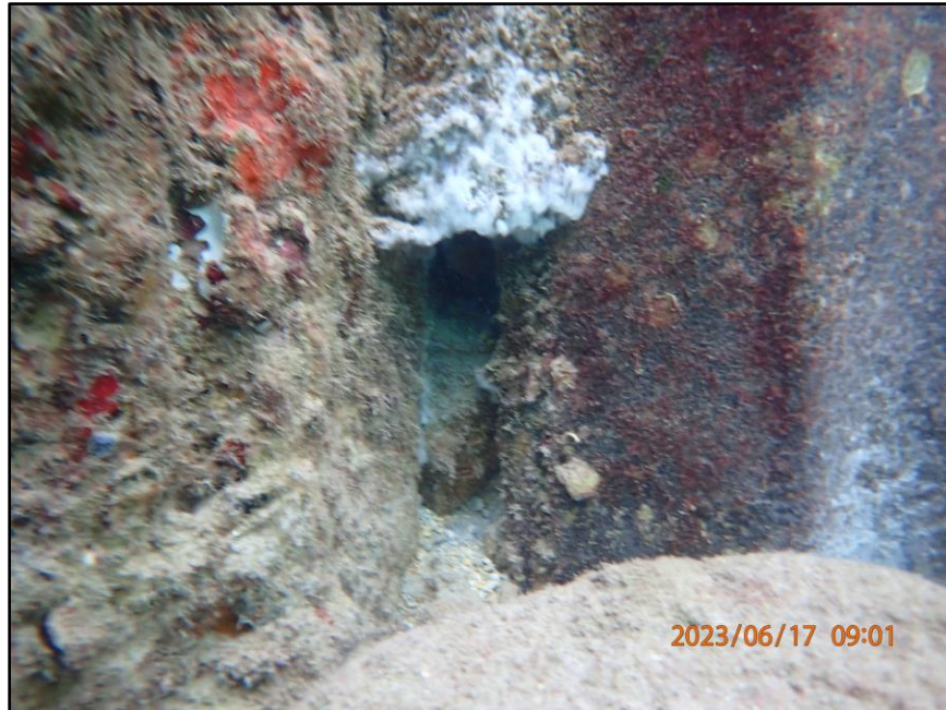
Photo 87: Void at bulkhead connection at mudline STA 4+70
