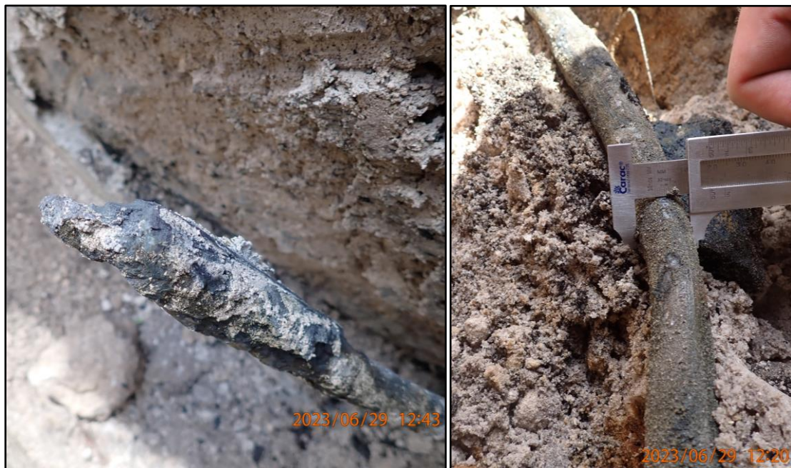
Photo 64: Section 5 Failed tie rod at STA. 2+75 E (left) and bent tie rod at STA. 0+05 E (right)
