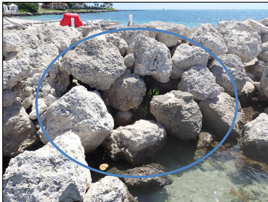
Photo 47: Section 2 localized riprap slope steeper than 1:1
