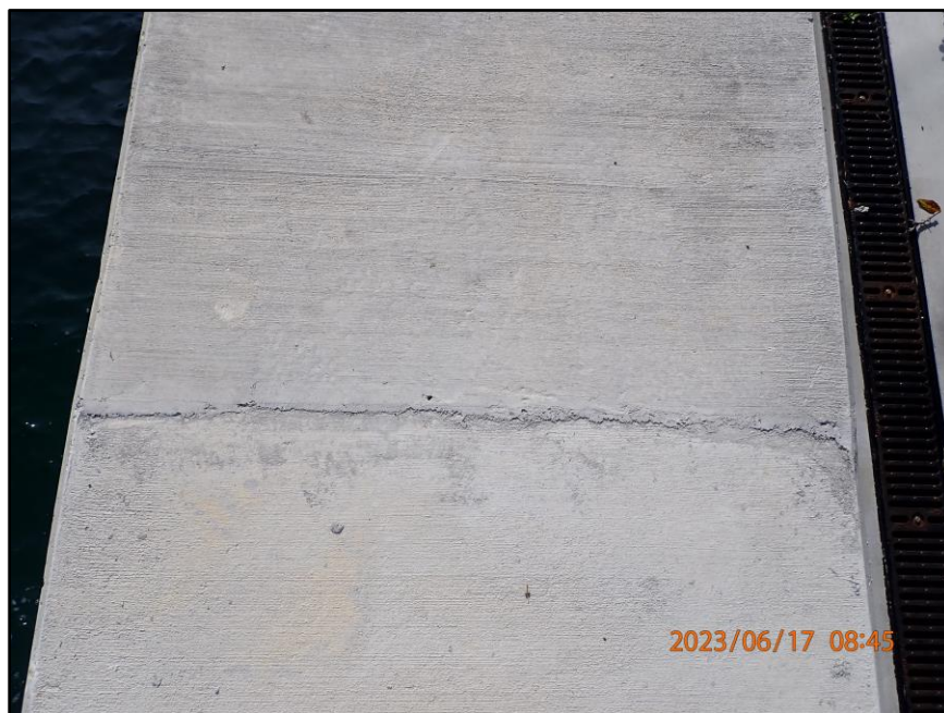
Photo 86: Localized shrinkage cracks
