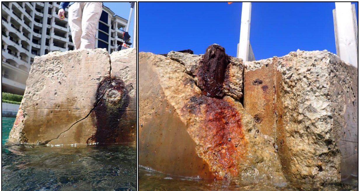
Photo 99: Intermittent severe cracking and spalling on offshore face due to severely corroded embedded cleats
