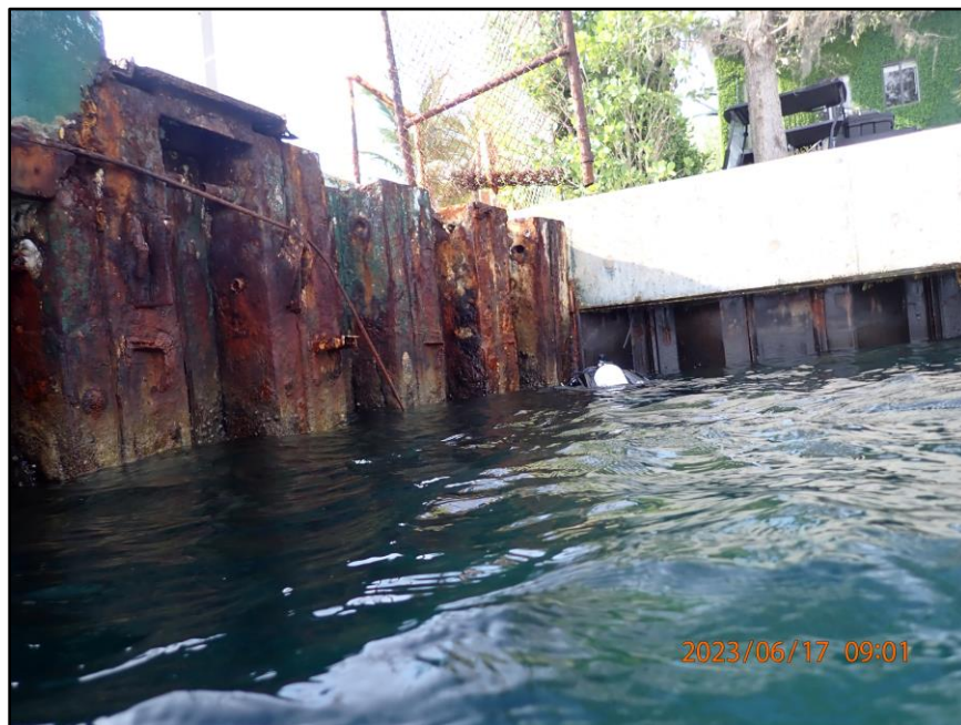
Photo 88: Failed cap from STA 4+70 to 4+90, severe corrosion of the steel sheet pile
