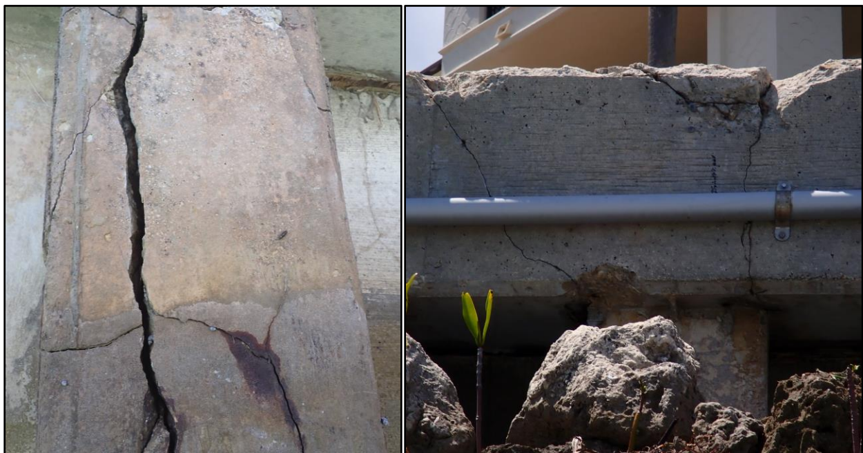
Photo 61: Section 5 Typical severe deterioration of concrete king piles with typical major deterioration of the concrete pile cap
