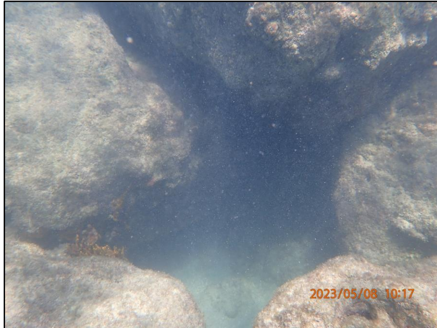
Photo 46: Section 2 localized moderate voids in the rip rap
