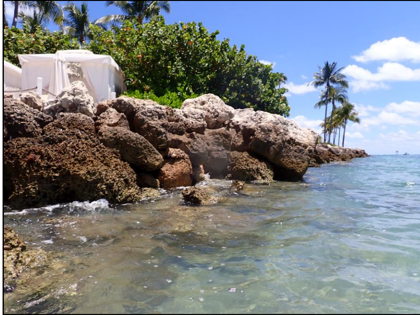
Photo 45: Localized 1:1 riprap slope at the western extent
