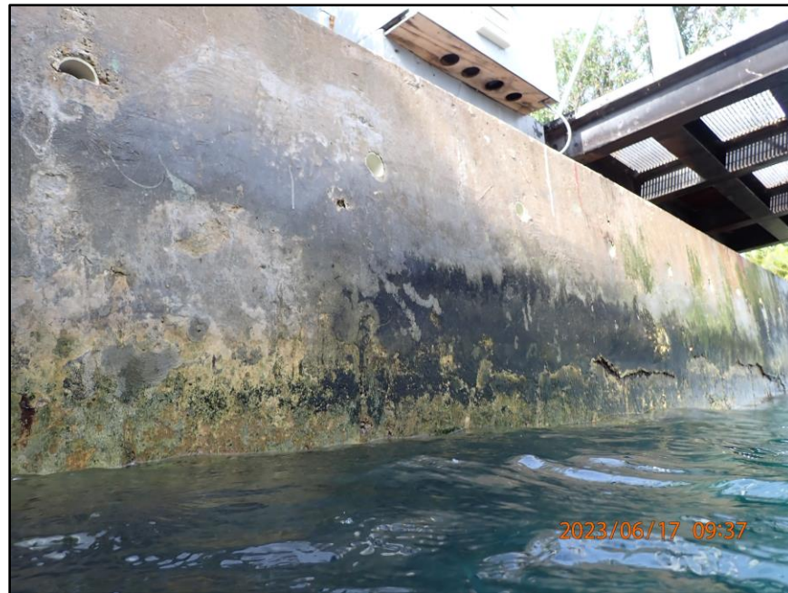
Photo 89: Intermittent delamination of the concrete cap STA 0+00 to STA 0+84
