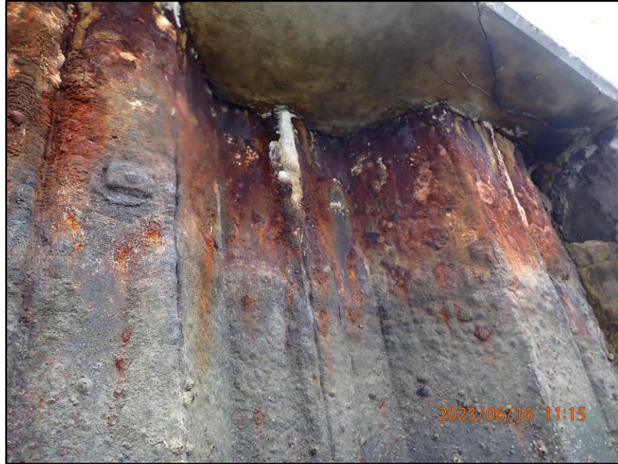
Photo 70: Typical condition of steel sheet pile and concrete cap
