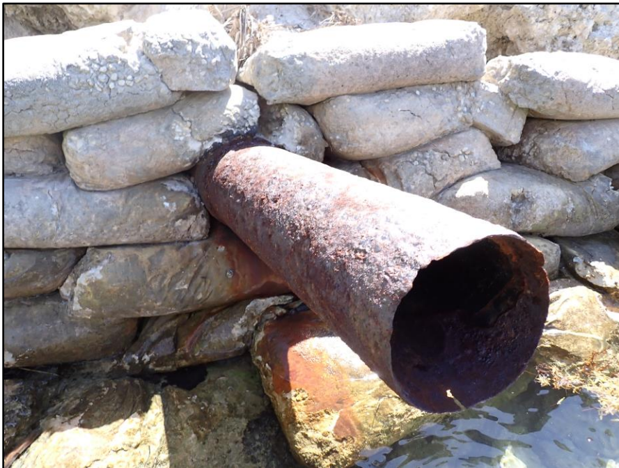
Photo 49: Section 2 severe corrosion of steel outfall
