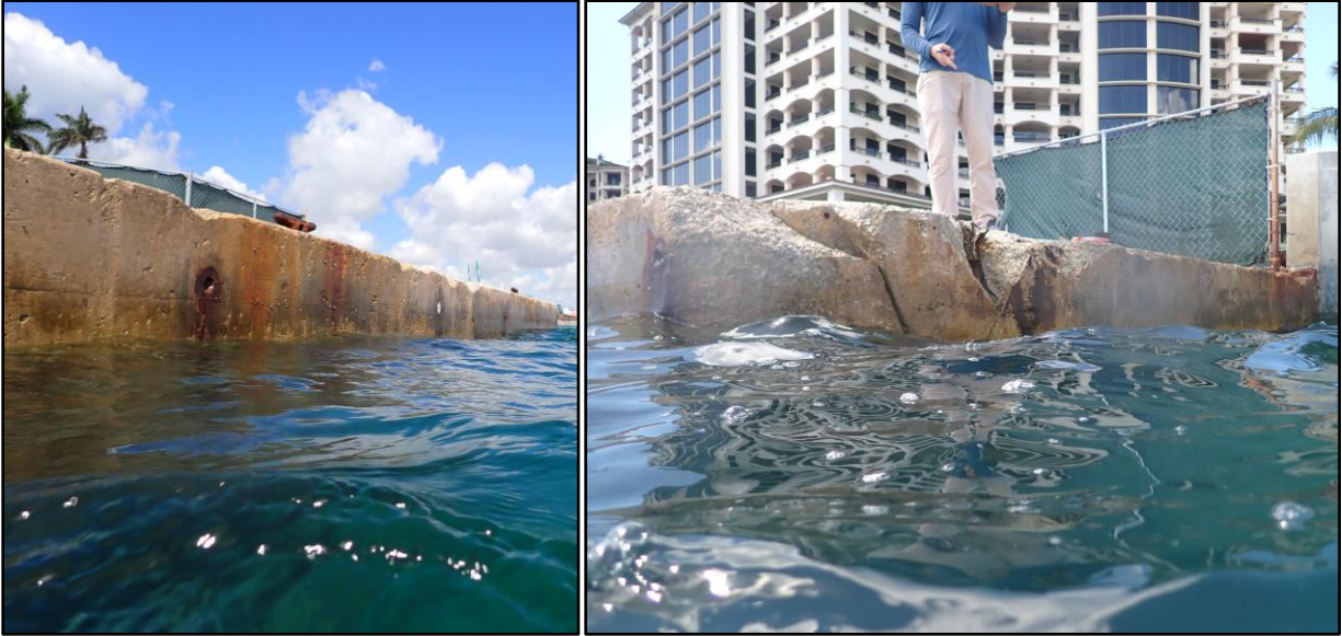
Photo 100: Typical widespread moderate erosion and spalling of the offshore face of the cap on the north face (left) and severe spalling of the cap on the west face (right)
