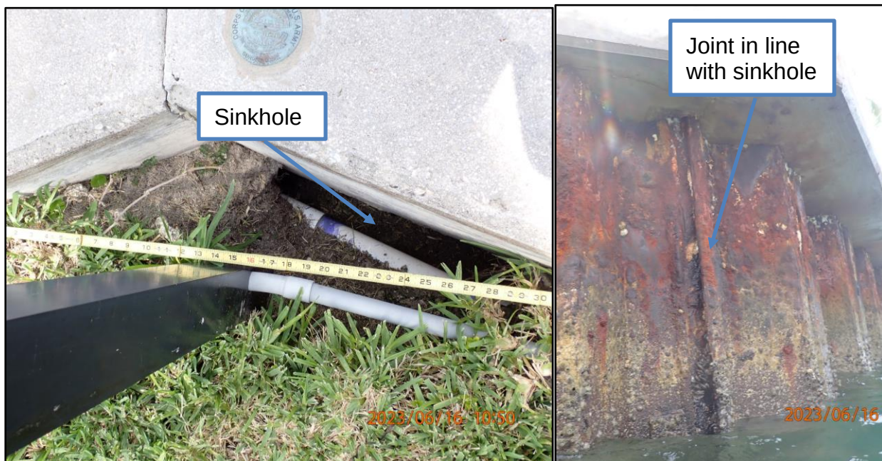
Photo 73: STA 12+18 Sinkhole and in line joint at corner of bulkhead
