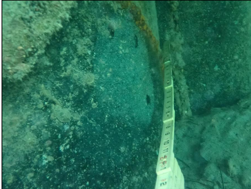
Photo 36: Section 12 View of new pipe pile portion of combi-wall through deterioration in original outer sheet
