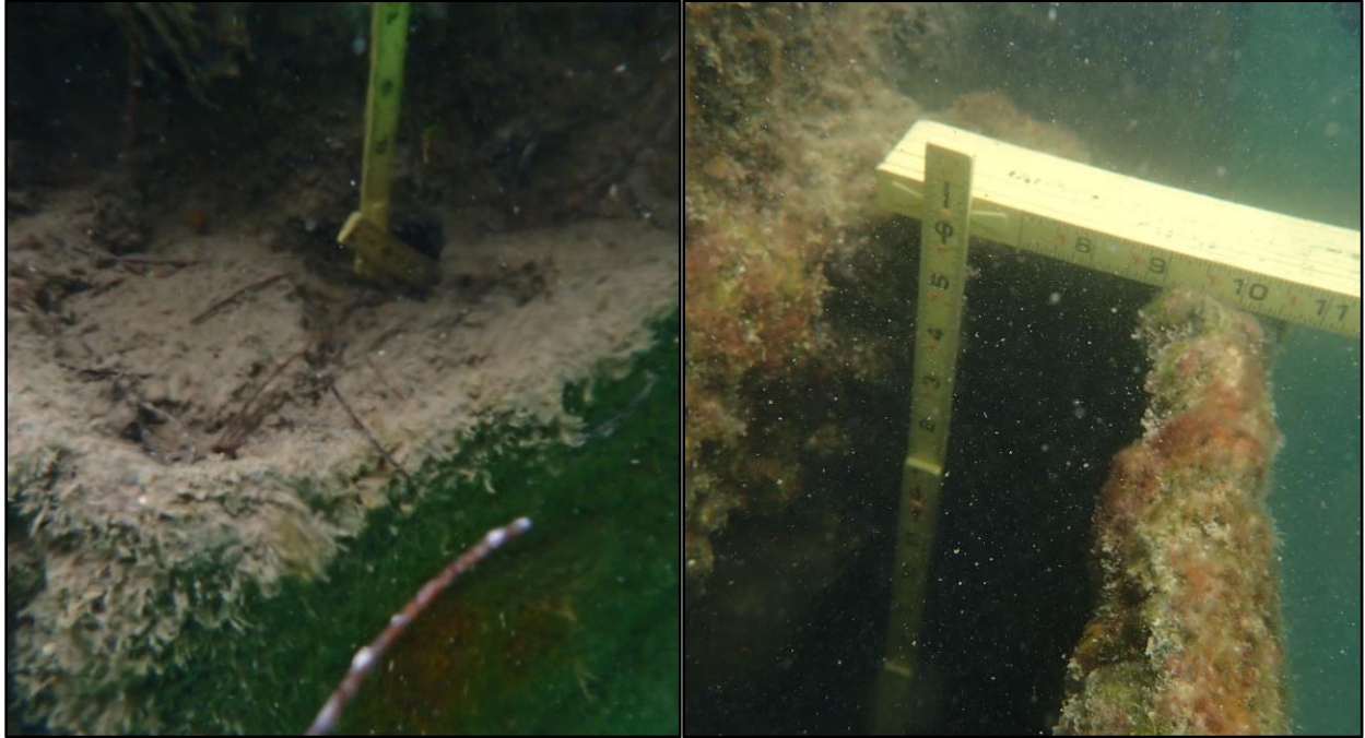
Photo 53: Voids in between the offshore edge of the Section 3 cap and the bulkhead
