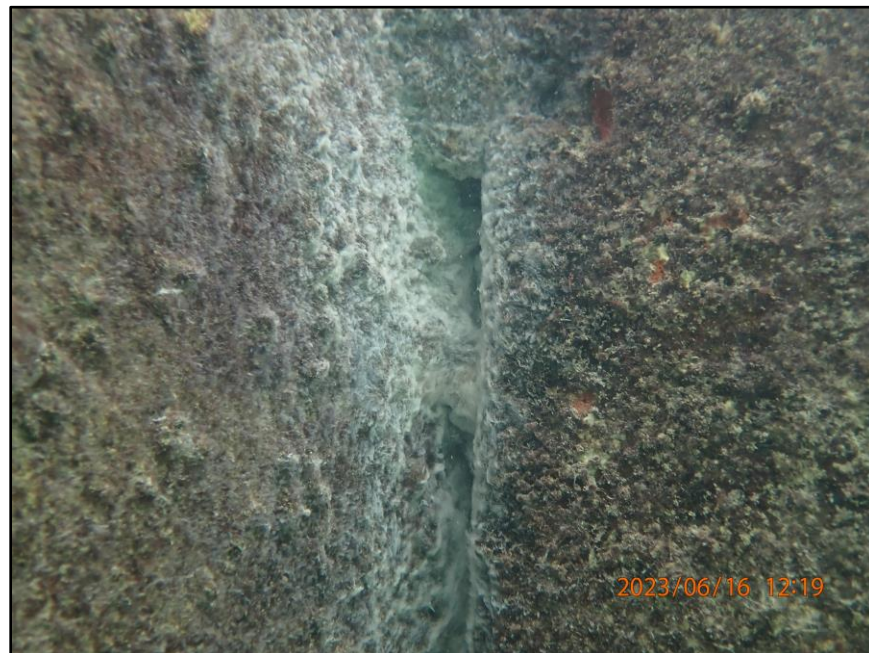
Photo 68: Typical evidence of freshwater intrusion at the pile panel interface
