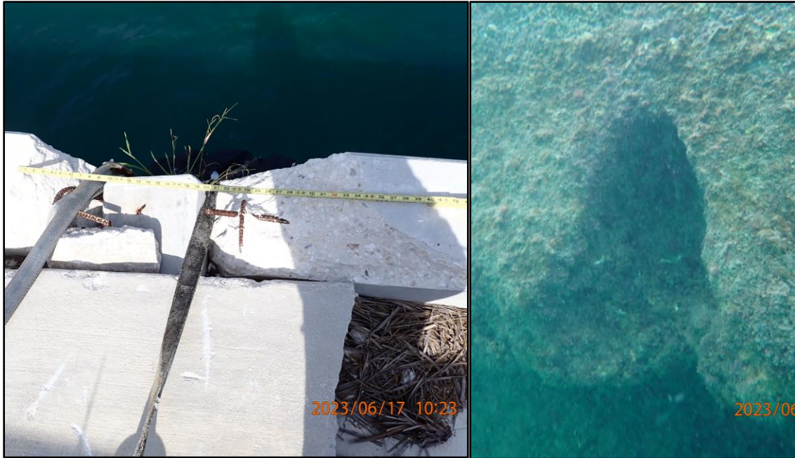
Photo 90: Widespread major to severe spalling of the concrete cap, STA 0+84 to STA 5+80
