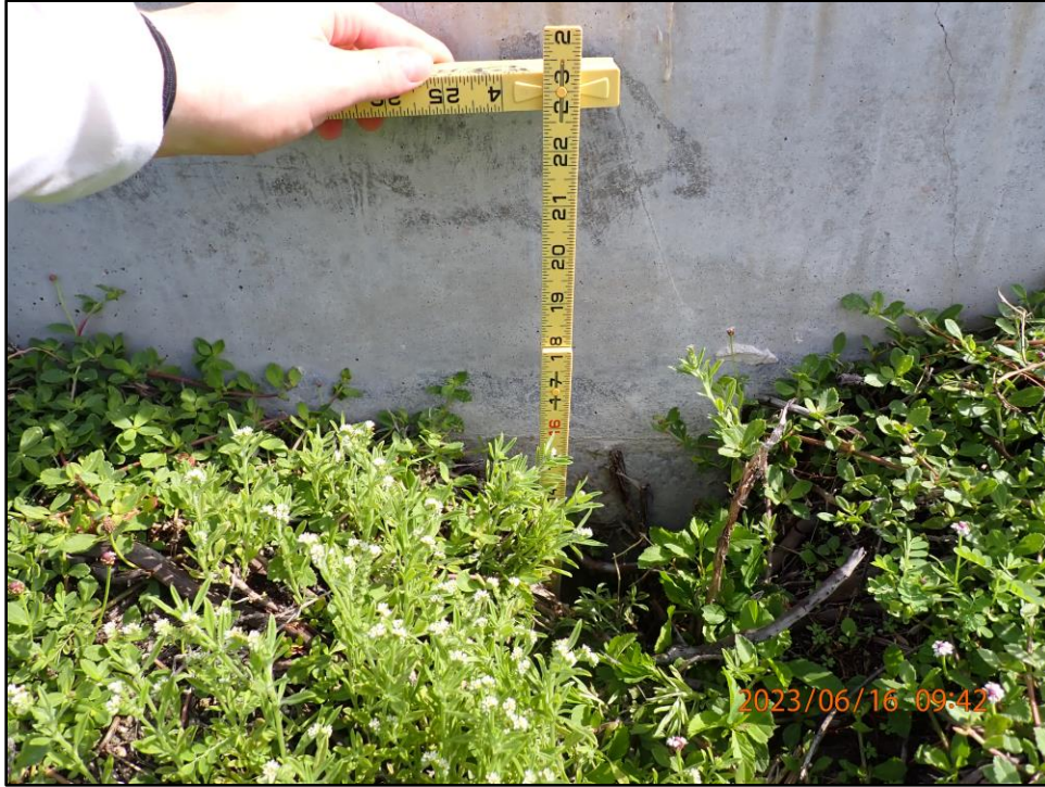
Photo 77: Typical view of Section 8 sinkhole
