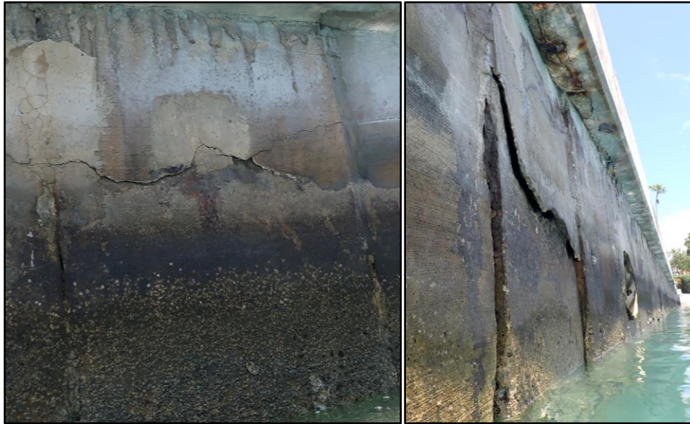
Photo 56: Widespread spalling and cracking of the Section 4 concrete sheet pile
