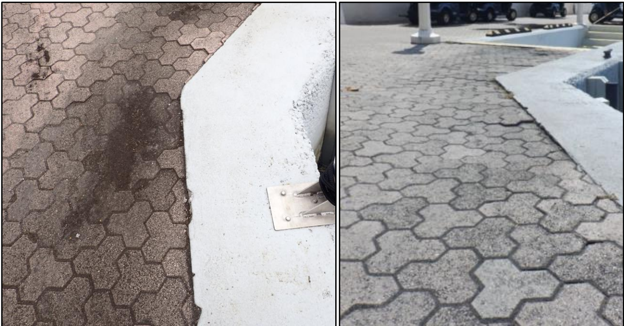
Photo 54: Minor settlement of the pavers STA 4+70, 2023 (left) and 2019 report (right)
