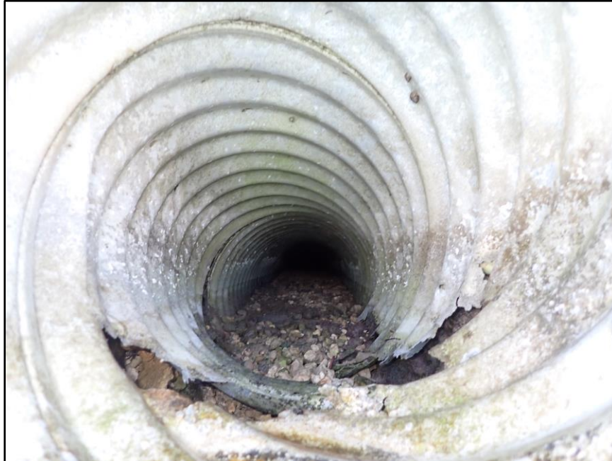
Photo 60: Section 4 STA. 0+30 Typical partial blockage of corrugated steel outfall with severe corrosion in the tidal zone
