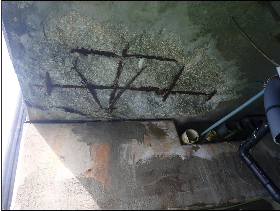
Photo 55: Severe spall in soffit slab adjacent to the Section 3 bulkhead termination
