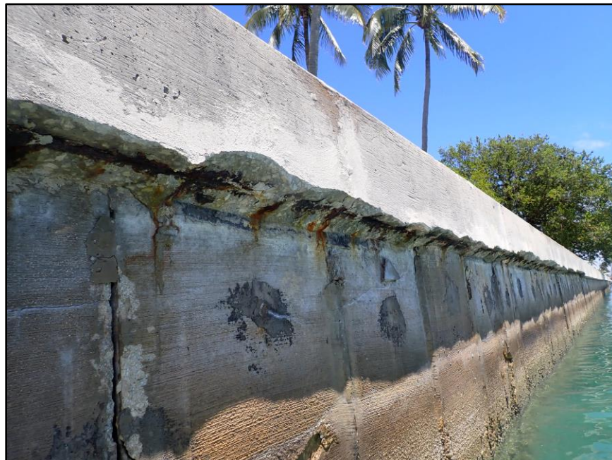
Photo 59: Severe spalling of Section 4 concrete cap with severe corrosion of the exposed reinforcement around STA 8+90.
