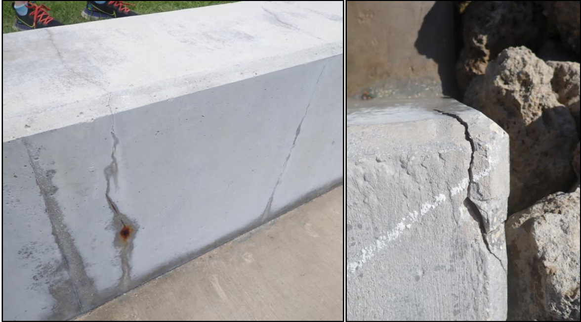
Photo 93: Intermittent cracking of the concrete cap up to 1/8 in. with localized cracking up to 1/4 in. forming a closed spall
