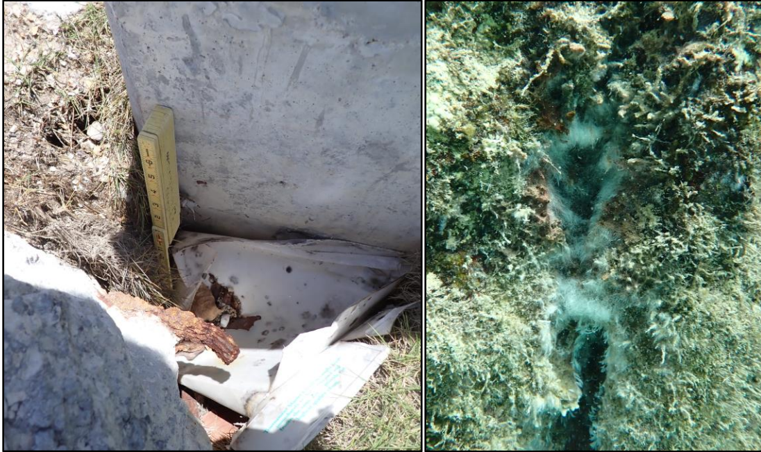
Photo 95: Sinkhole at northeastern termination (STA 2+90) with signs of freshwater intrusion visible at the in-water portion of the joint
