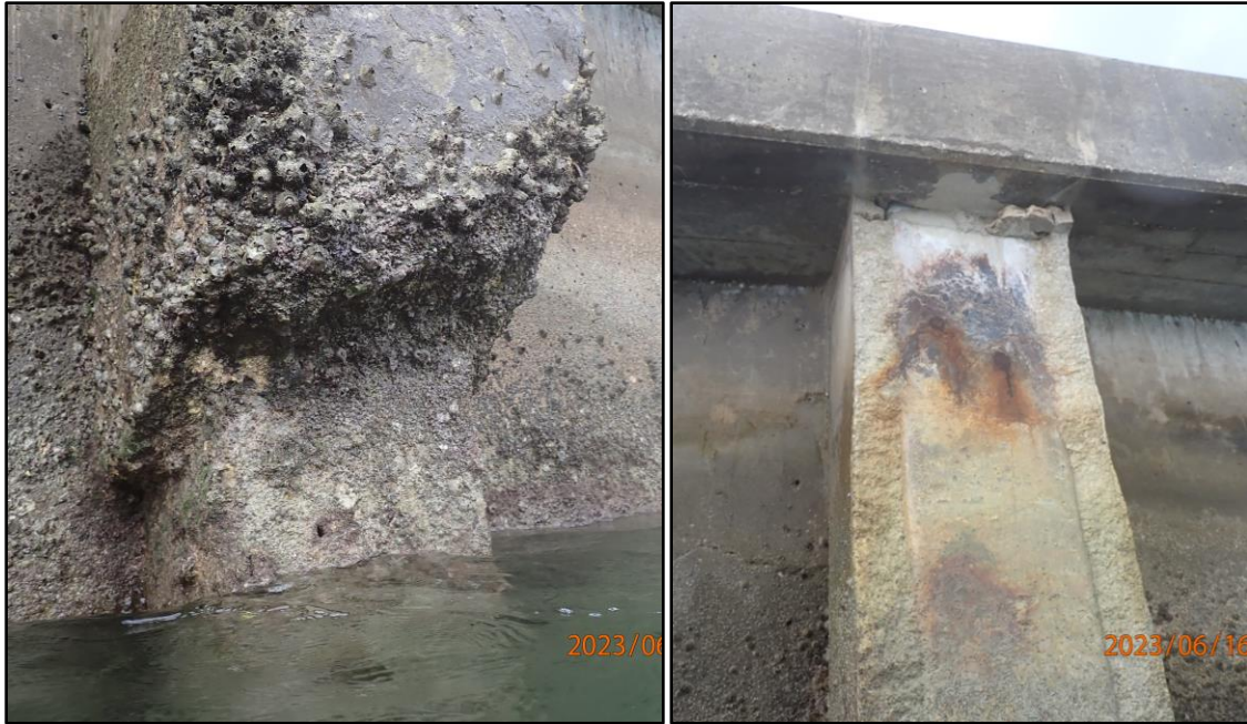
Photo 65: Typical washout of concrete pile encasement (left) and localized delamination of offshore extent of pile encasement
