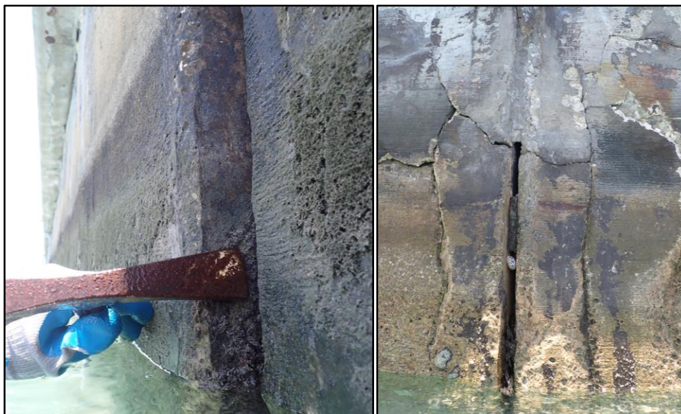
Photo 57: Section 4 STA. 5+72 Typical view of lateral separation (left) and horizontal separation (right) at sheet pile joints
