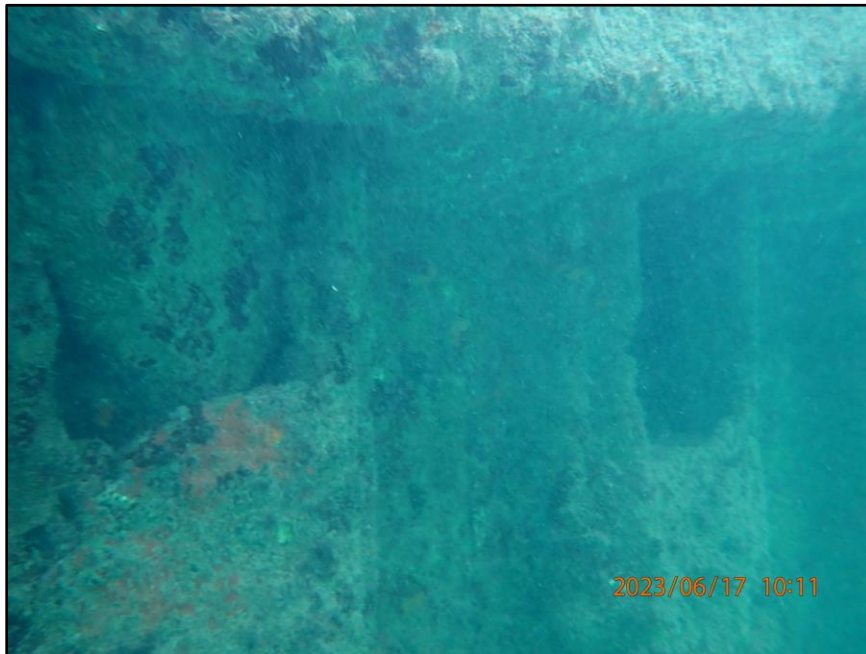
Photo 32: Derelict bulkhead steel sheet piles visible within Section 11 ferry basin
