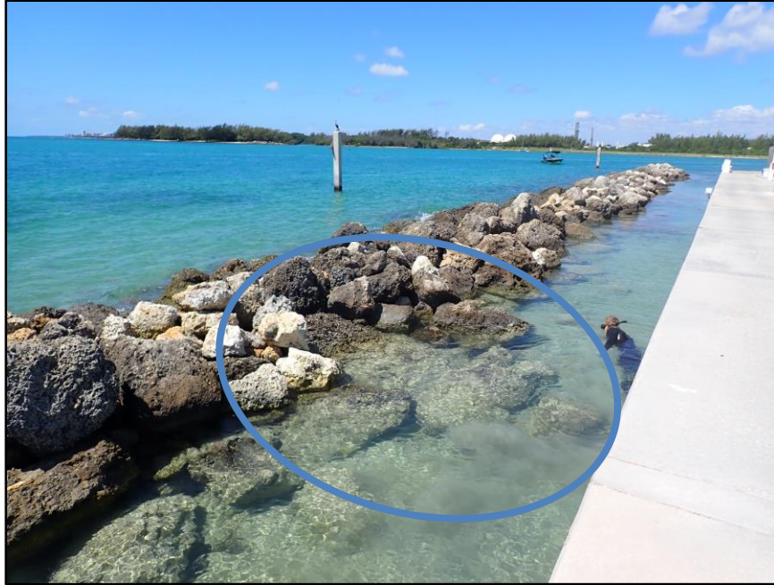
Photo 48: Section 2 riprap shifted downward STA 0+55, facing northeast
